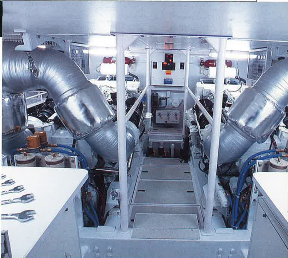
The 72's engine room looks like that of a much larger yacht. The space has six-foot-plus headroom.
